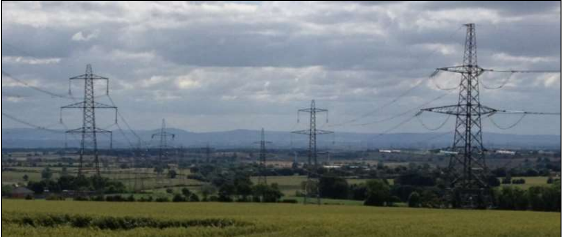
Figure 5.4 Suspension Tower (left) and Tension Tower (right)
